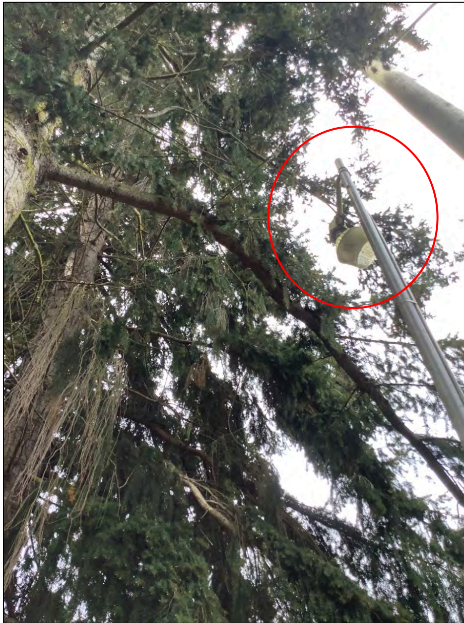
Photo 13: Note broken streetlight near Tree 2 (circled in red).
